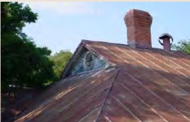
Roof materials in San Antonio's historic districts are diverse. Barrel-rolled clay tiles (top) and standing seam metal (bottom) are just two examples. (Photos: Ron Bauml, San Antonio Conservation Society)
