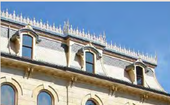
Decorative metal cresting adds to the character of this building and should be preserved. (Photo: Ron Bauml, San Antonio Conservation Society)
