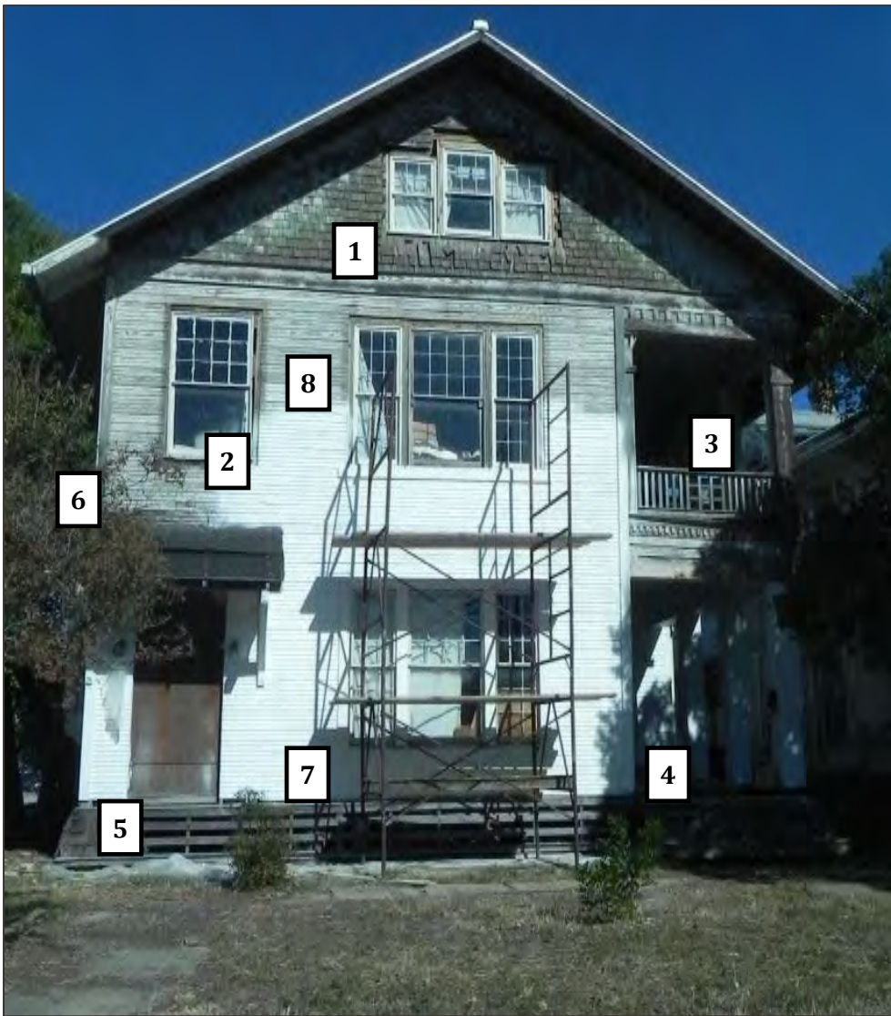
Through an extensive rehabilitation effort, the structural and visual integrity of this historic structure will be recovered.
