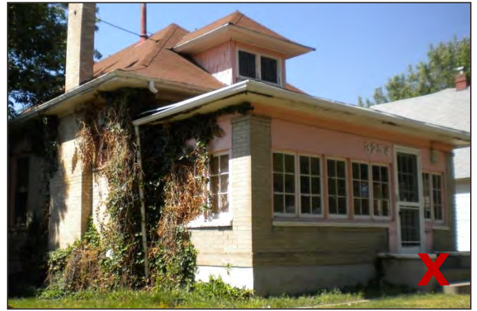
The enclosure of this front porch significantly alters the historic character of the building.
