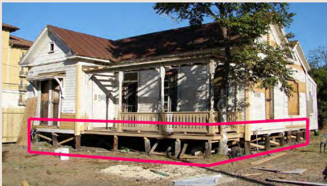
Pier and beam foundations—both concrete (top) and cedar (bottom) are common in San Antonio. (Photos: Ron Bauml, San Antonio Conservation Society)
