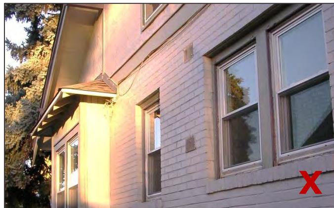
Do not use replacement windows, such as these vinyl inserts, that do not match the historic character of the building's original windows.
