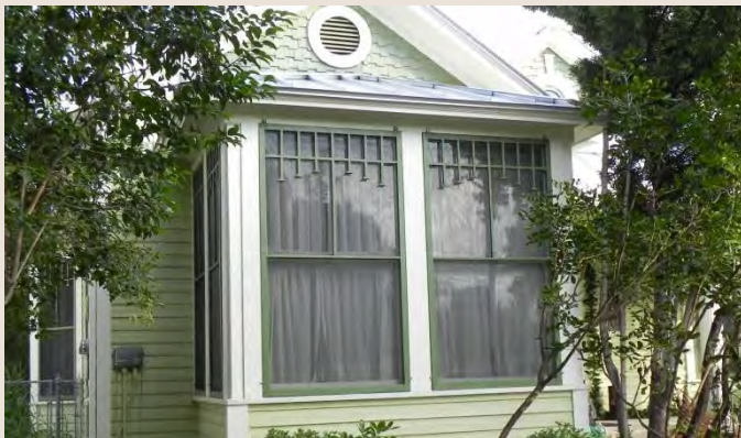
These historic window screens are unique in design and contribute significantly to the character of the building.
