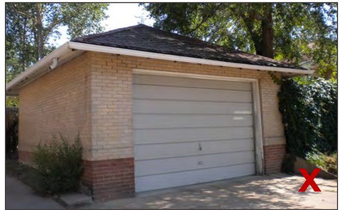
A metal replacement garage door is not historically accurate and distracts from the character of this historic garage.
