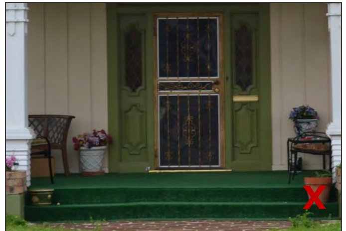
Covering porches with tile or synthetic coverings like this turf can trap moisture and can lead to deterioration.
