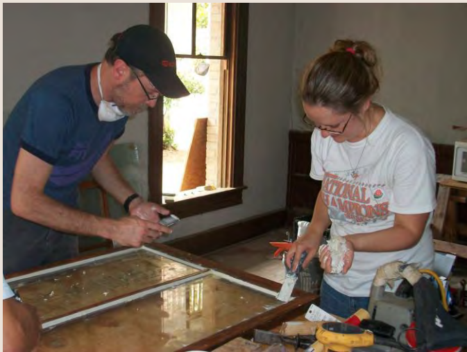
Applying glazing putty to historic windows helps make them weather tight reducing heat loss and gain.
