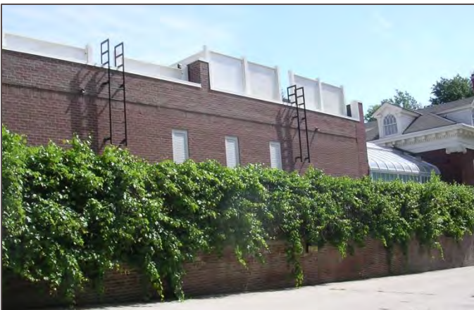
Rooftop mechanical equipment on this addition to a historic structure is screened from the public right-of-way.
