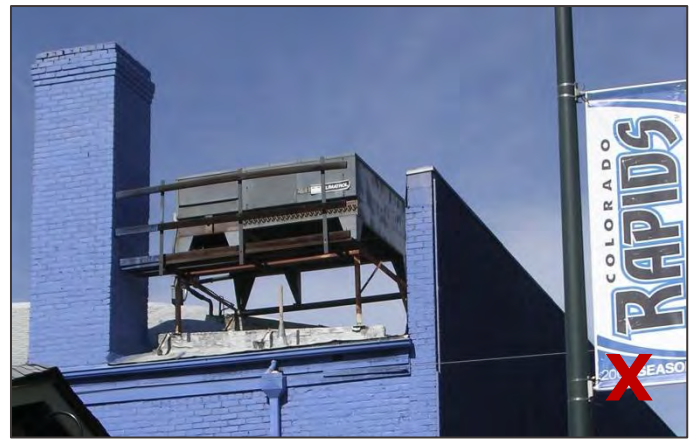
Rooftop mechanical equipment should not be visible from the public right-of-way.
