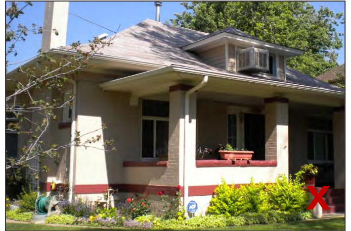
Air conditioning units should not be placed on the primary façade of historic structures.
