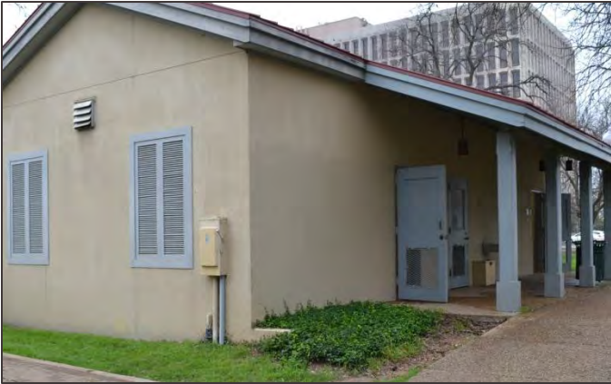
This utility box is located on a secondary façade and painted to match the color of the primary historic structure.
