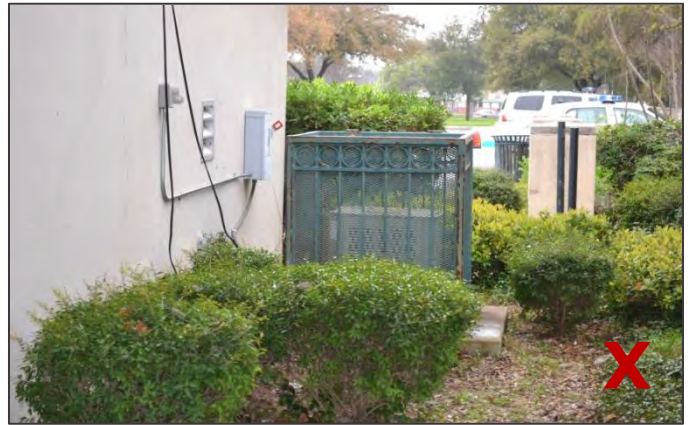
While the air conditioning unit is screened from view, the wall mounted utility box and other wires do not match the color of the building and distract from the overall character.
