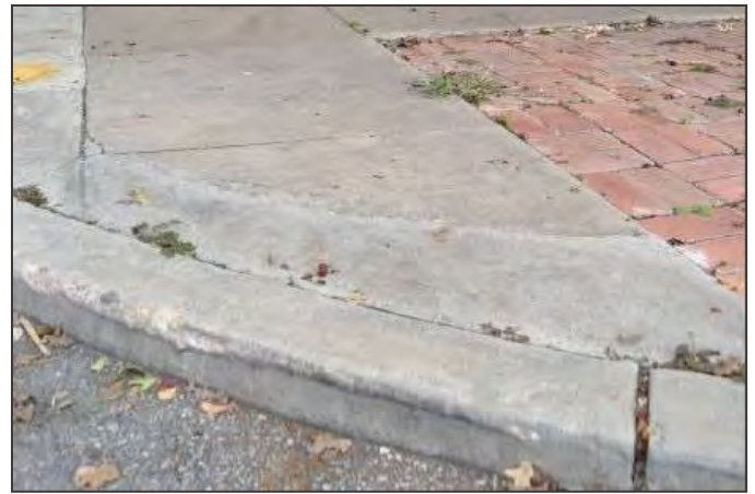
Intersection of concrete and brick sidewalks at W. Woodlawn Avenue and Howard Street.
