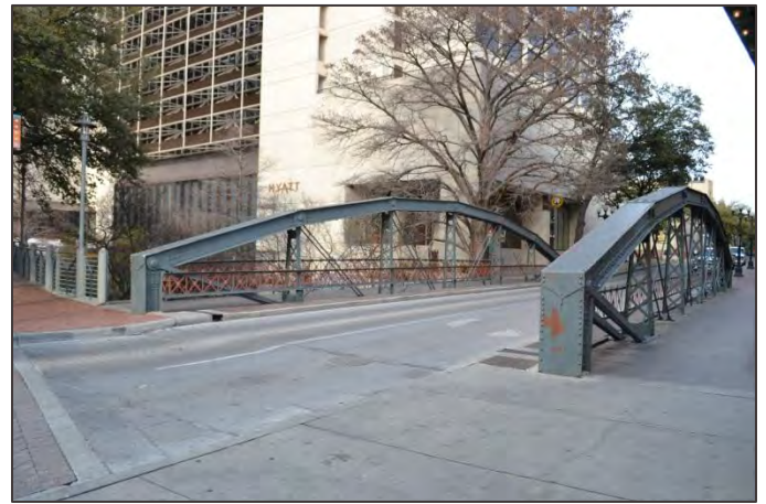
Bridge over the River Walk at E. Crockett St., Alamo Plaza Historic District.
