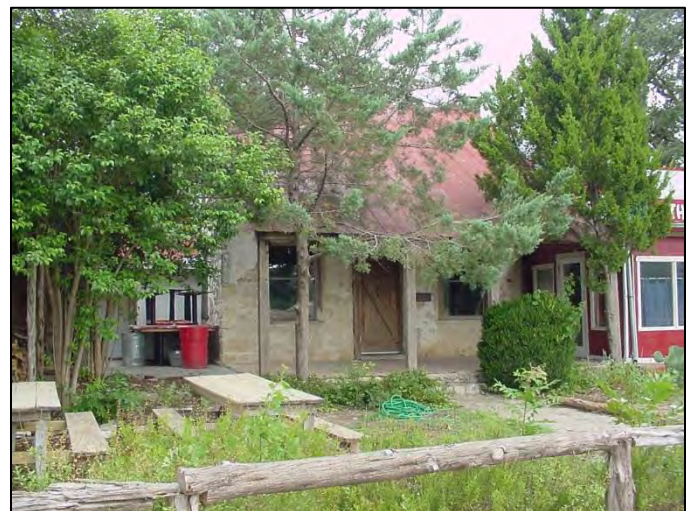
Stone house, Leon Springs Historic District. Note that the one-story addition at the right is non-historic.
